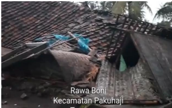
Figure 2. Houses in Pakuhaji Sub-district were damaged by a tornado on Monday (1/2/2021)
