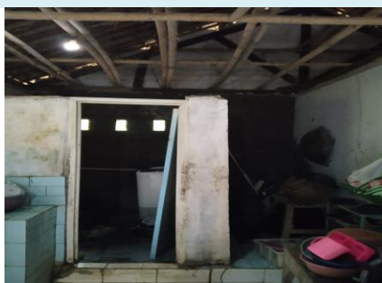
The condition of the room in the house is damaged due to the fragile roof structure.
