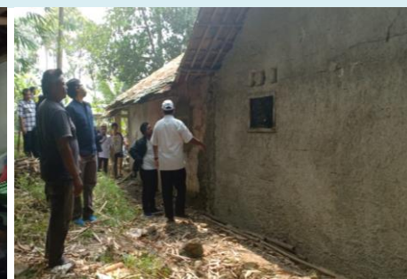
No column reinforcement, so it is very prone to collapse.
