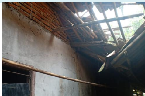
Roof construction is made of rotting bamboo. It has collapsed when a big wind hits it.
