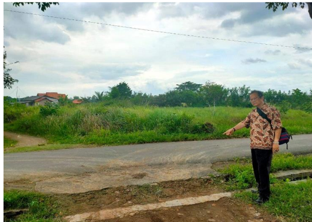
3. Environmental Road Damage
